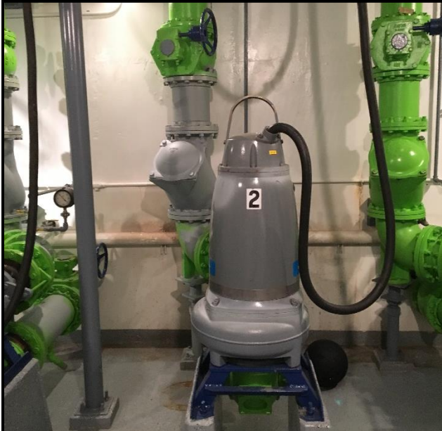
Lift Station No. 17 Pump
